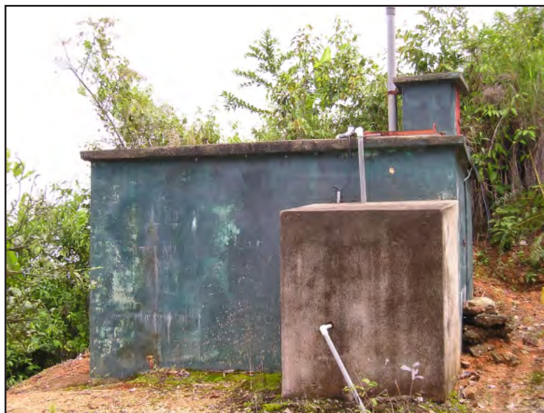
Figure 3. A storage tank built by one community's local ASADA. Water from a nearby stream is piped to this holding tank where chlorine is used to disinfect the water before it is distributed to households
